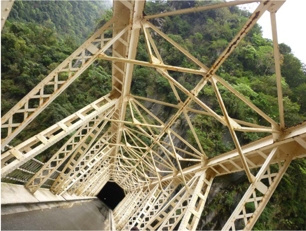
Imagine the structural stress and strain
